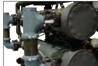
Evaporator manifold terminated in victaulic coupling.
